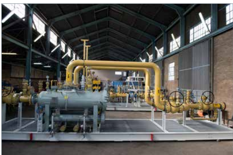
The plant has been designed to be fuelled by any one of three fuel sources, that is, natural gas, distillate fuel or light crude oil.
