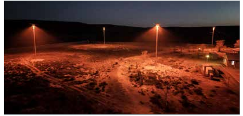
Solar highmast lighting solution at the Sutherland Community Health Centre, complying to the unique requirements of the Sutherland Central Astronomy Advantage Area lighting standards.
