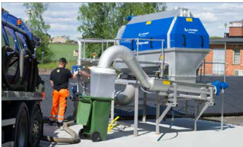
The Lackeby Roto-Sieve® with extended lifting pipe and bag system in use at Broby WWTP waste water treatment plant in Sweden.
